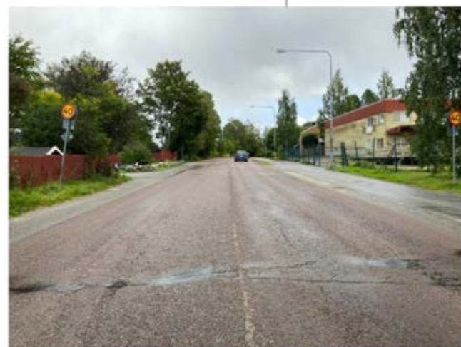
Pictures of Bölevägen and its surroundings. There are a narrow or no sidewalk at the north side of the street, (Photo: Eva Maaherra Lövheim, 2021).
